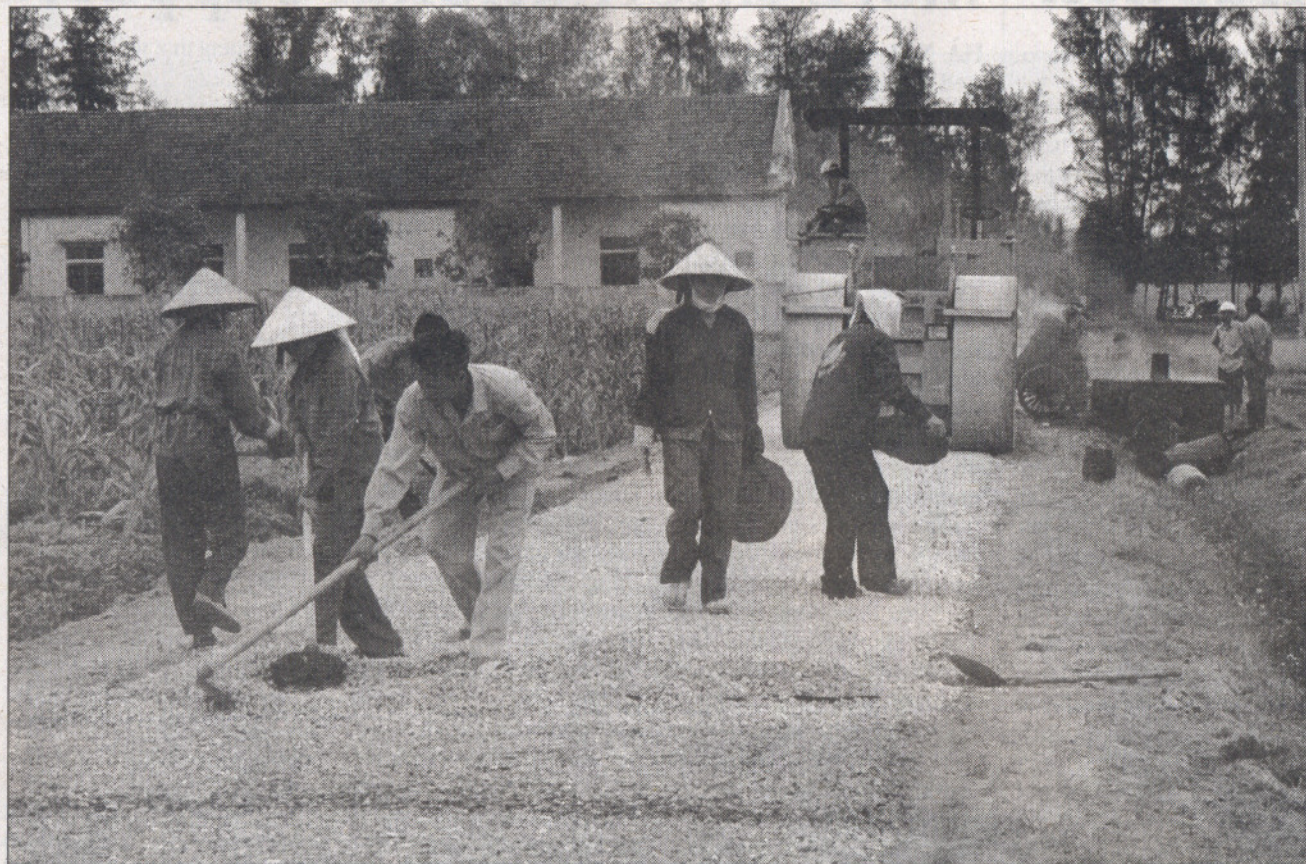
Workers upgrade a road in Nghi Liên Commune, Nghi Lộc District in Nghệ An Province. A project on training provincial road engineers aims to improve the design, construction and maintenance of rural roads in provinces across the nation. — VNA/VNS Photo Lan Xuân
