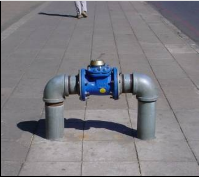
An exposed water meter in the path of pedestrians
