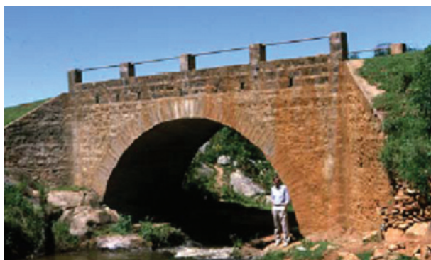
Figure 8.56 Completed masonry arch bridge with splayed wing walls on hard rock foundations
