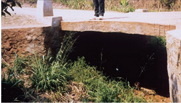
Figure 10.3 Box culvert partially blocked by vegetation
