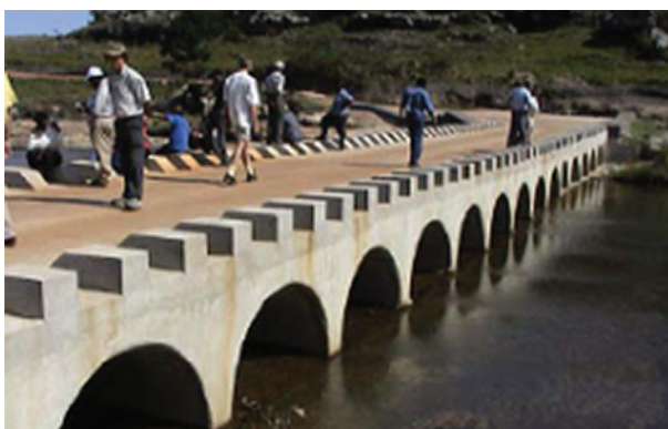
Figure 8.62 Raised kerbs on a vented causeway allow water to pass over the structure with minimum disturbance, but provide protection from vehicles driving off the structure.
