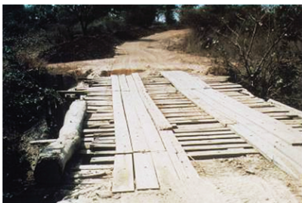
Figure 8.57 Timber deck with floor planking and edge beams in need of repair
