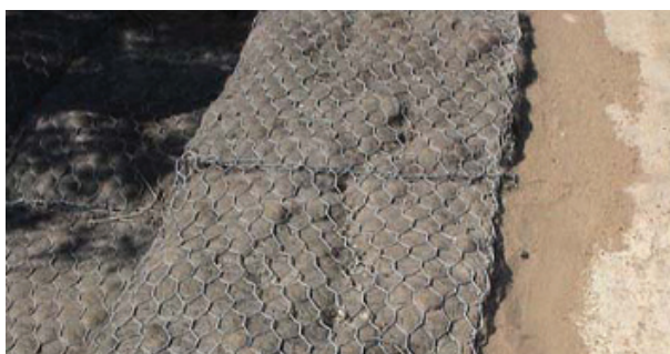
Figure 8.9 Natural fibre matting inserted in the top and face of the gabion can encourage vegetation growth to stabilise the gabion face and retained material.
