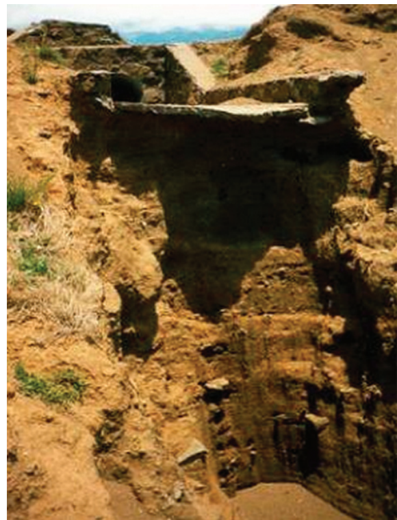
Figure 8.39 Severe erosion at outfall
