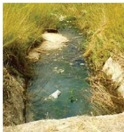
Figure 8.14 Ponding in outfall channel
