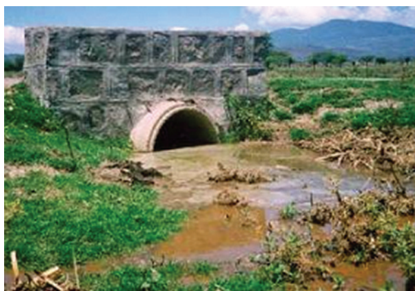
Figure 8.13 Ponding at culvert outfall
