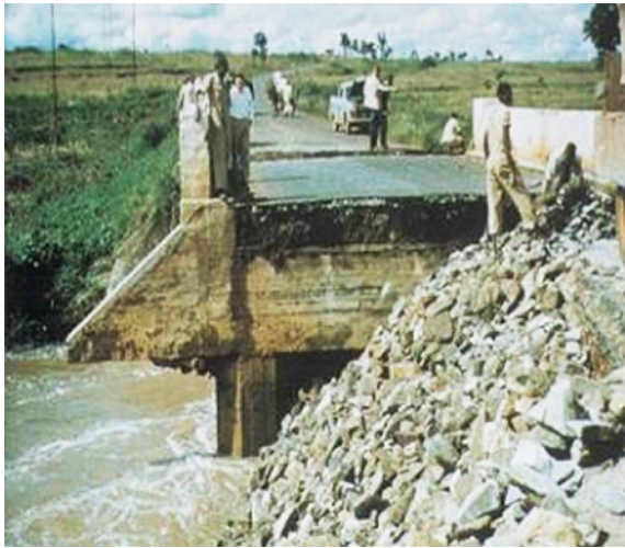
Figure 8.1 Bridge damage due to scour of abutment
