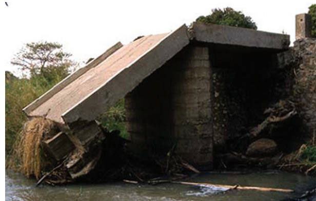
Figure 8.3 Failure of structure due to a combination of constriction of the watercourse (structure too small), scour and inadequate protection of abutments.
