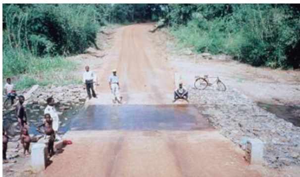
Figure 8.6 Concrete slab drift
