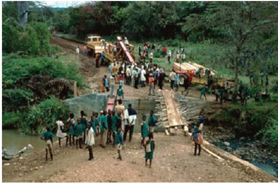
Figure 7.33 - Steel beams being moved into position using labour methods without the use of cranes ready for completion with a timber deck
