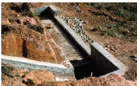
Figure 7.53 - Flow spreader structure at the outlet of a mitre drain on a steep fragile slope. Bio-engineering planting should be established downhill of such structures.
