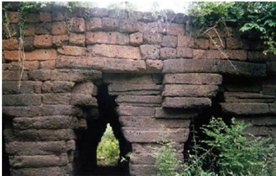
Figure 7.1 Dry jointed, multiple opening, cantilevered laterite stone culvert approximately 1,000 years old and still in service.
