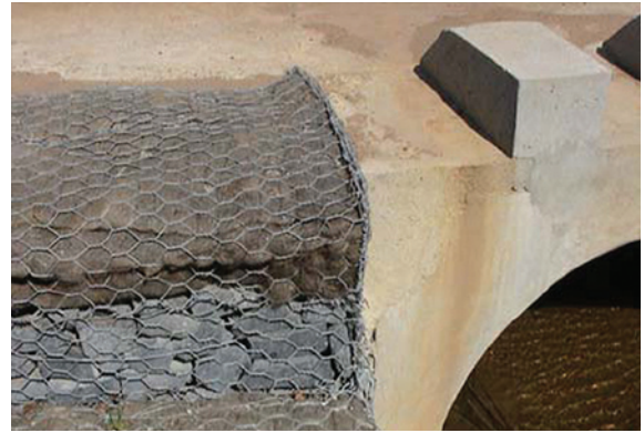
Figure 7.23 Natural fibre matting inserted in gabion protection works to encourage rapid growth of vegetation cover
