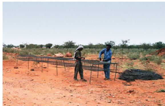
Figure 7.48 Steel reinforcement cage being assembled for the cut-off wall in a drift
