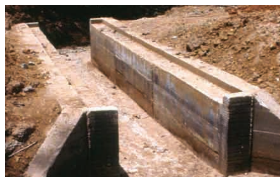
Figure 7.54 - A simple reinforced concrete walled box culvert ready to receive pre-cast top slab units (timber or reinforced concrete).
