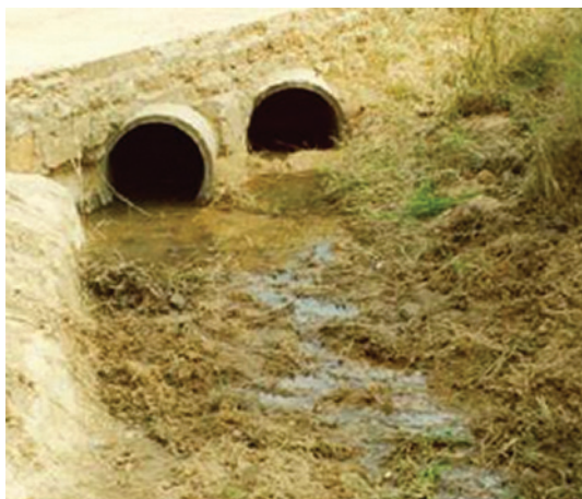
Figure 5.7 Ponding at culvert outlet
