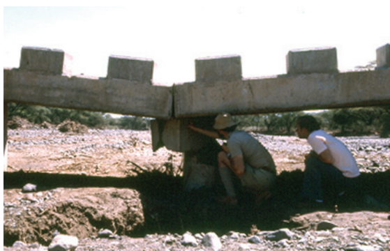
Figure 5.4 Collapse due to settlement
