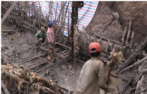
Figure 5.5 Timber piles being driven into very soft ground for a culvert foundation (requires specialist expertise not covered by this guideline)
