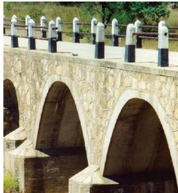
Figure 3.6 Pedestrian guard rails (in need of repair)
