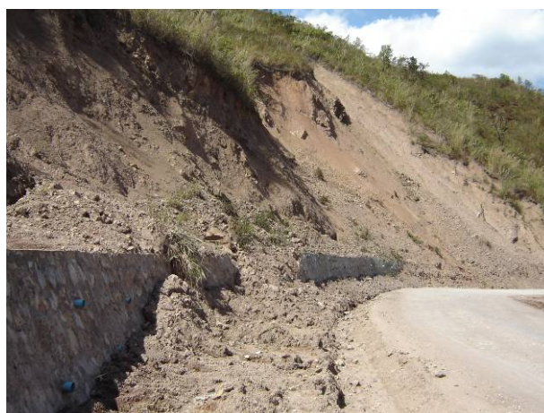
Figure 2-11: Failure of mortared masonry wall due to large scale slope movement
