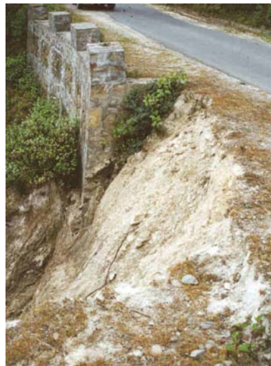
Figure 4-13: Erosion adjacent to wall
