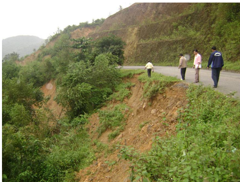
Figure 2-5: Fill slope failure
