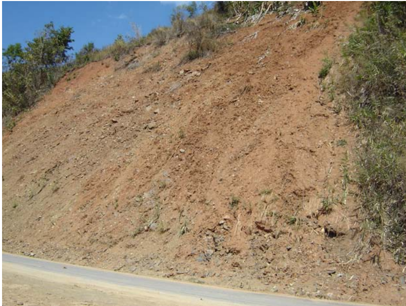
Figure 2-7: Typical slope erosion
