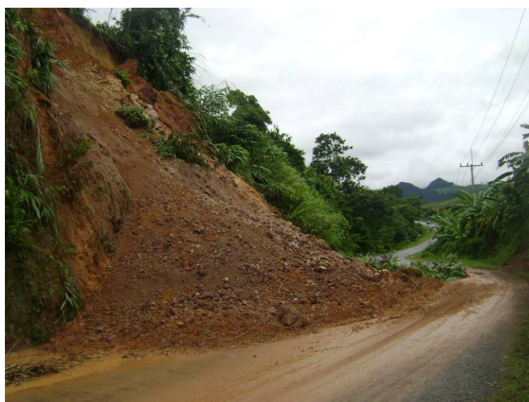
Figure 2-4: Failure of an over-steep cut slope
