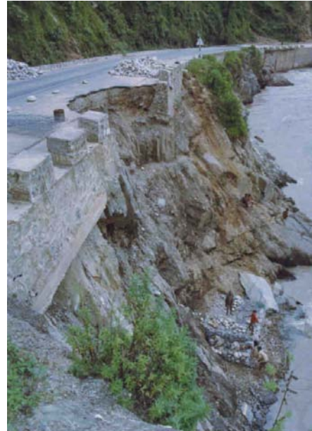
Figure 2-13: Masonry wall failure due to scour 1
