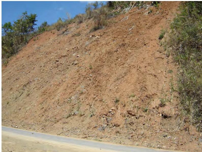
Figure 2-7: Typical slope erosion
