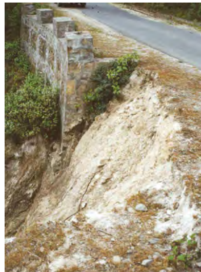
Figure 4-13: Erosion adjacent to wall
