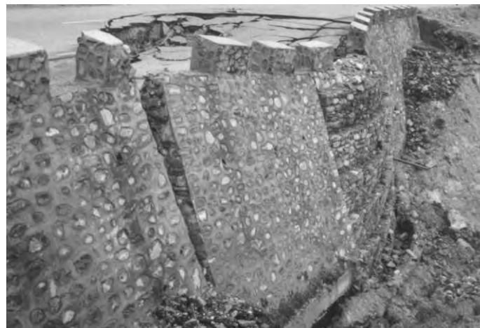
Figure 2-14: Failure following river flooding in front of wall 1
