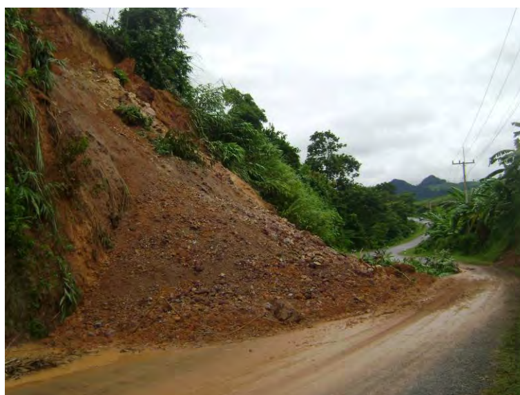
Figure 2-4: Failure of an over-steep cut slope
