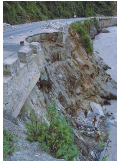
Figure 2-13: Masonry wall failure due to scour 1
