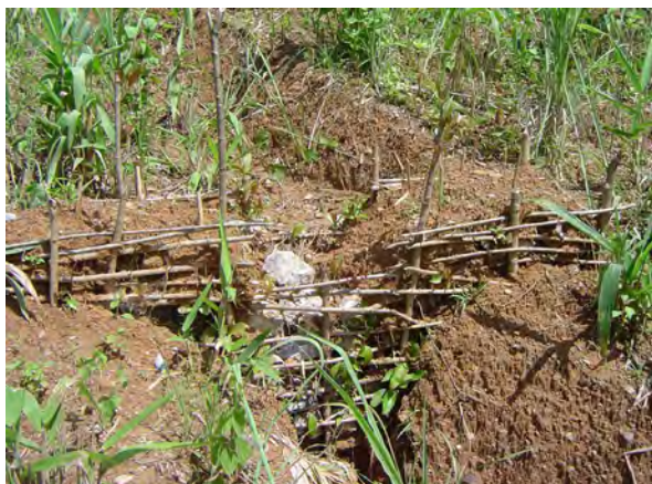
Figure 6-13: A live check dam on a soil slope, about 2 months after completion
