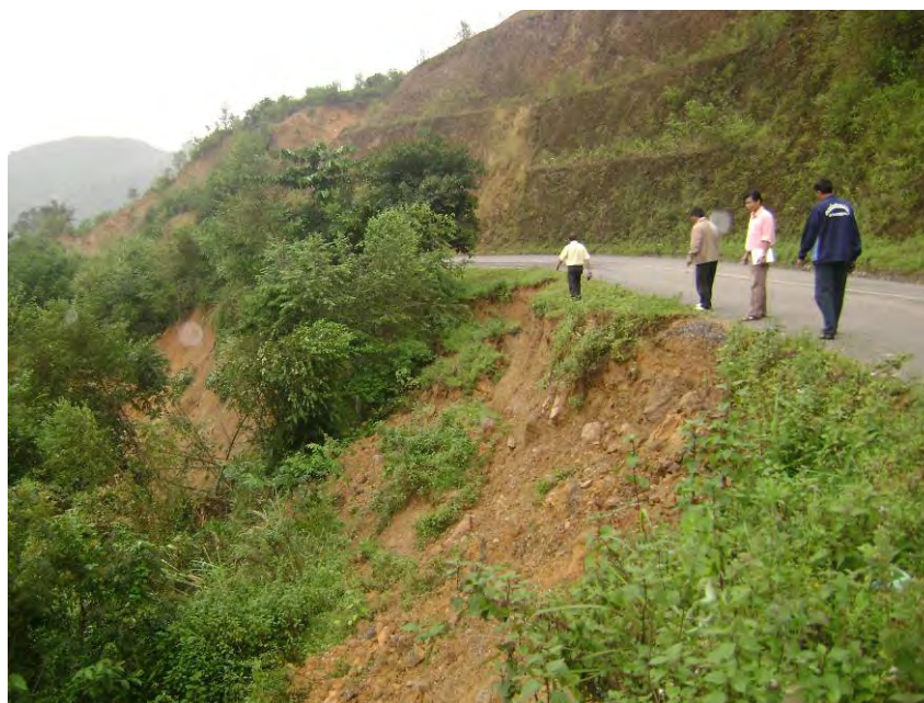
Figure 2-5: Fill slope failure
