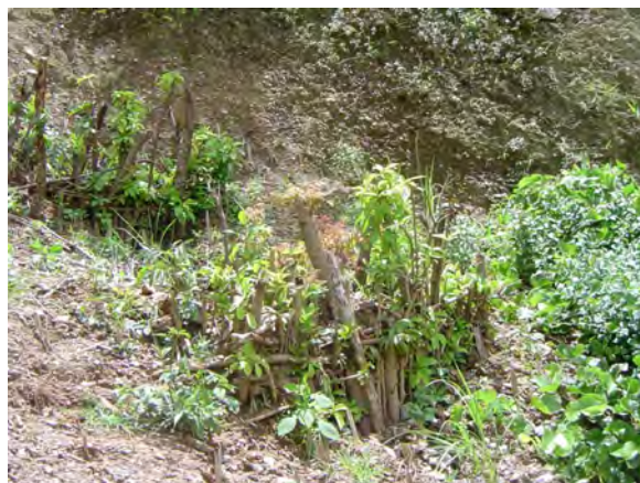
Figure 6-14: Live check dams about 3 months after completion, on a mixed debris slope
