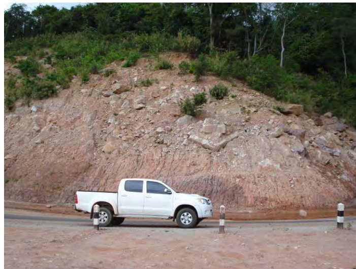
Figure 2-3: Shallow translational failure in colluvium
