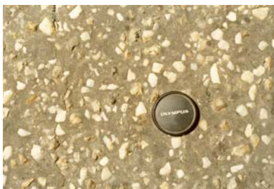
Example of a double Otta seal (using decomposed granite) plus after 10 years in service in a harsh, semi-arid environment with practically no maintenance.
