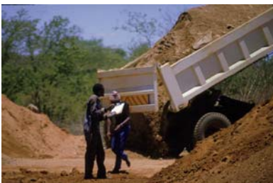
Good management procedures that prevents rejection of material on the road creates confidence in the quality assurance system and greatly reduces the risk of shortcuts and poor practice.
