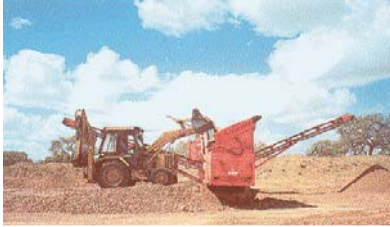
The operational characteristics of the Otta seal are such as to allow the use of as-dug natural gravel which can be screened, if necessary, to remove fines and over-size material.
