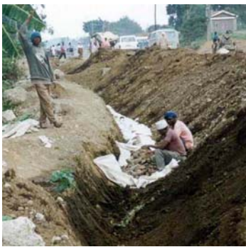
Construction of filter drains is well suited for labour based methods. Geotextiles used for filter drains should be of a type that does not get blocked by fines from surrounding soils.
