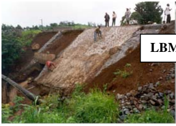
Inadequate culvert capacity, particularly in combination with high embankment, can result in severe damage and expensive remedial works.
