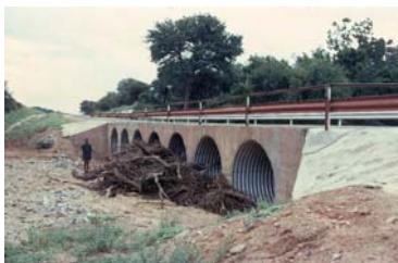
Banks of pipe profiles culverts are prone to blockage by trees even when large sizes are used.
