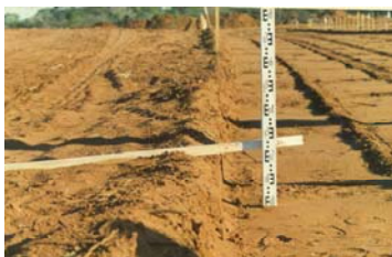
Collapse settlement in excess of 150 mm after impact rolling.
