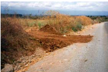
It is important to create an awareness amongst the public so that actions that lead to impaired drainage of the pavement can be prevented.
