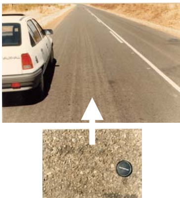
Loss of second seal due to bitumen hardening and embrittlement.
