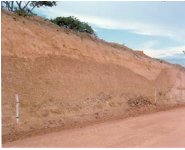
Laterite is a typical example of a “non-standard” material that has been successfully used in LVSR construction despite its non-compliance with traditional strength and plasticity requirements.
