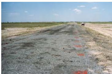
An example of severe distress to a runway surfacing due to salt attack resulting in damage within two years of its construction.
