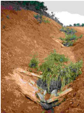
Concrete scour checks in side drain.
