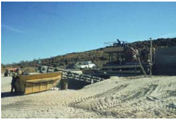
A small, simple crushing/ screening plant can be combined with labour adapted tractor operations.
