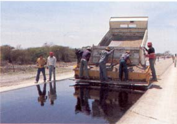
A typical surface treatment operation – spraying a thin layer of bitumen onto a road surface prior to the application of a layer (s) of aggregate.
