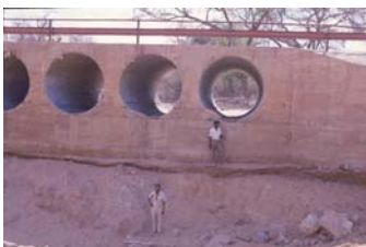
When there is a risk of erosion at outlets, suitable aprons and other protective measures are required.
