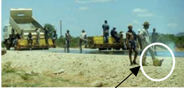
Having spray cans with bitumen emulsion available at all times during surfacing operations for repairing minor faults is part of good quality assurance.
