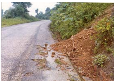
Road surfacing failures due to blocked side drains
