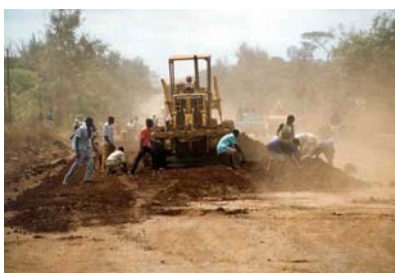
In most cases, the removal of over-size material is best carried out by the use of manual labour.
