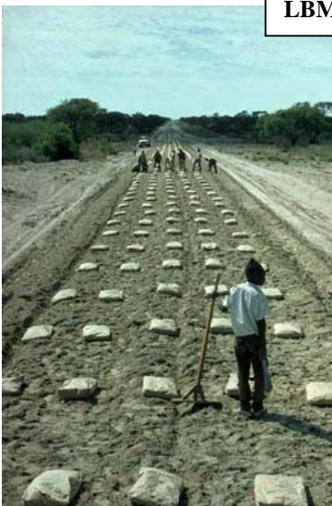
Stabilisation with lime or cement can be successfully applied with basic methods and use of manual labour.
