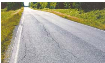
Typical longitudinal cracking and pavement deformation caused by large volumetric changes of an expansive soil subgrade.
