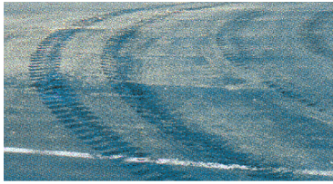
Heavy braking and tight cornering situations require an appropriate choice of high stability surfacings. Asphaltic concrete and possibly Cape or double Otta seals would be preferred to sand, slurry, chip or single Otta seals.
