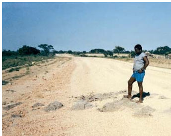
Burrowing animals such as termites can cause damage to pavement layers unless nests are removed properly and poisoned with an approved pesticide during clearing and grubbing.
