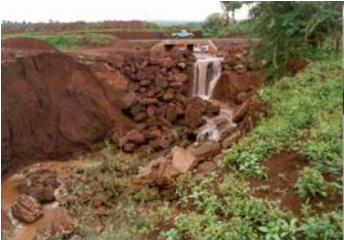
Erosion in outlet channels can cause considerable environmental damage in sensitive areas.
