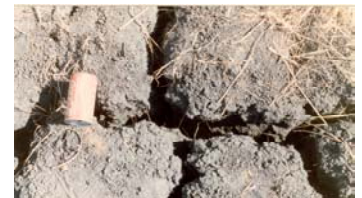
Expansive “black cotton” soil exhibiting wide-spaced shrinkage cracks.
