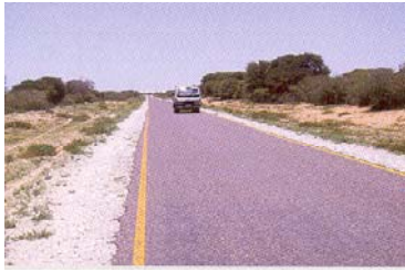
An example of a single Otta seal with a sand cover performing very satisfactorily after more than 13 years in service and without any surfacing maintenance in a harsh environment.
