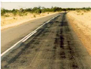
Bleeding due to embedment of surfacing aggregate in base.
