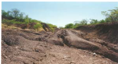
Eroded subsoils on borrow floor bed – susceptibility to erosion leads to siltation in water courses.
