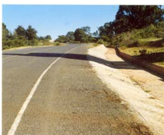
Good sight distances on a well-designed LVSR. Note wide shoulder and shallow slope to drainage ditch which both reduce potential hazards.
