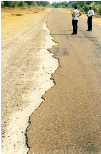
Severe edge break on a 5 m carriageway even at relatively low traffic levels (< 100 vpd).
