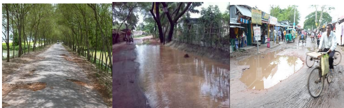
Figure 7.7.2: Condition of road on the different points of the study area
