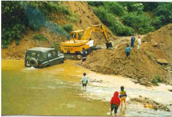
Figure 64 - Landslide caused by rainfall
