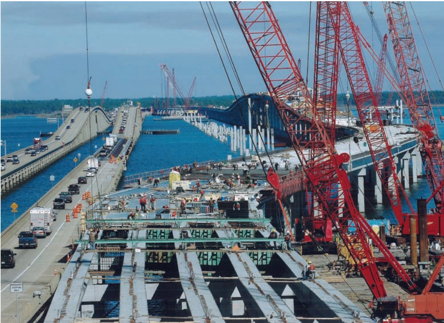
Quick action by the Florida DOT and FHWA enabled replacement of the I-10 Escambia Bay Bridge on an accelerated schedule after it was destroyed in a 2004 hurricane.
