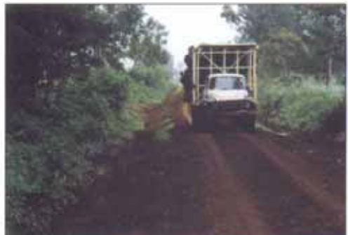
Traffic able to use Reshaped Roads Shortly after Rain
