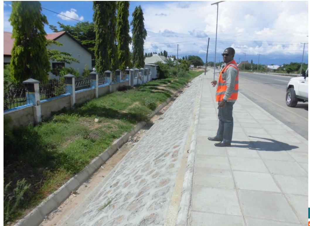
Side drains, pedestrian walk ways and embankment protection at CH. 0+00 of Emmaus-Arican Dream Rd
