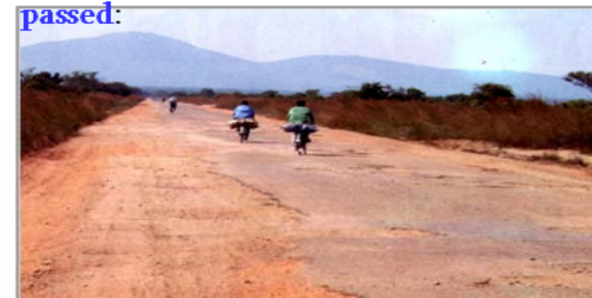
A new road surface, a new base and a new drainage has become necessary (Need for Rehabilitation).
