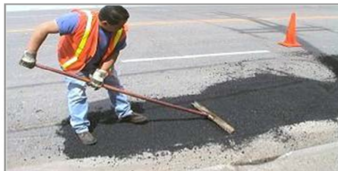
Pothole patching is needed permanently.
