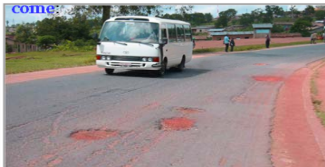
A complete new road surface is needed now.
