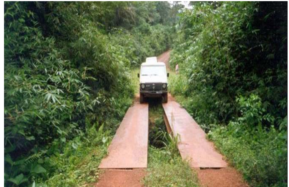
Bailey Bridge system for Rural Roads in Kindu / East Congo (GTZ Project) (Two double T-steel beams covered by iron plate for each lane)
