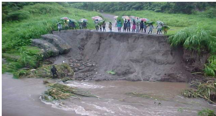
Typical Bougainville Coastal Trunk Road washout after heavy rain
