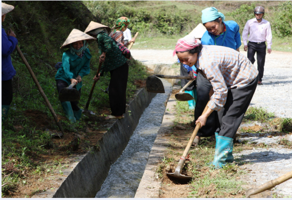
A construction crew upgrades the road between Lai Chau and Lao Cai towns, northern Vietnam.
