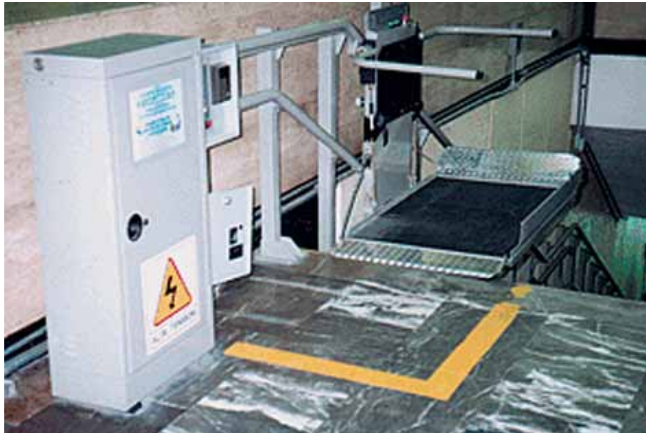
Figure 3.58 Stair lift used in the Mexico City Metro
