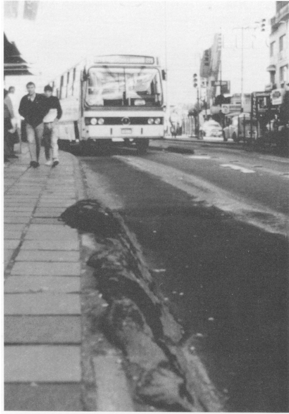
Plate 14 Pavement creep along a busway
