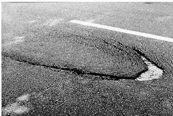
Cracking outside wheeltracks – parabolic crack
