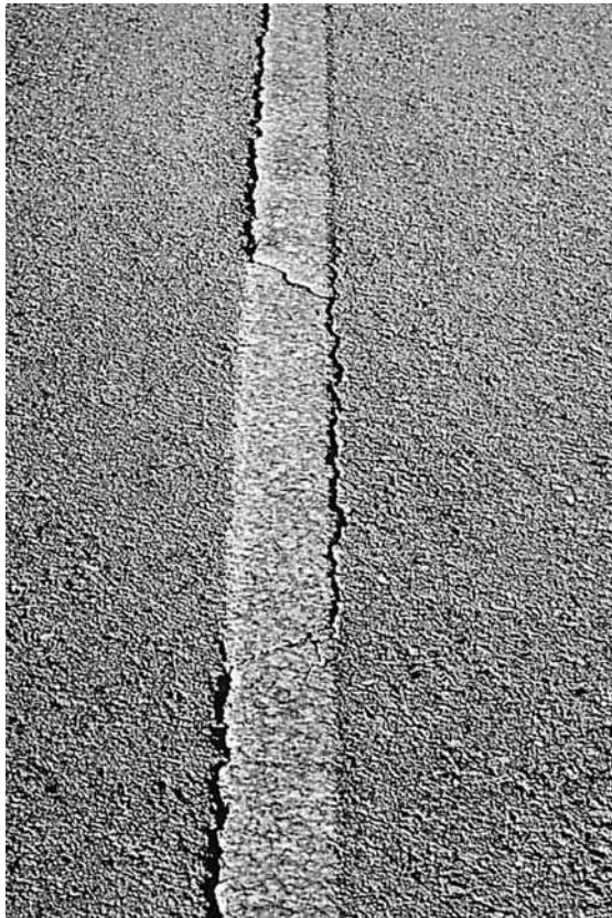
Cracking outside wheeltracks – along white line
