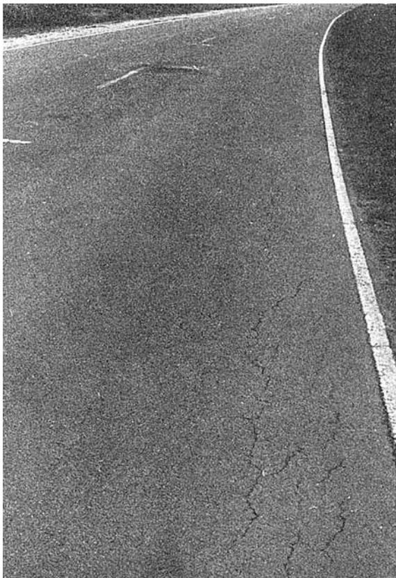
Cracking in wheeltracks
