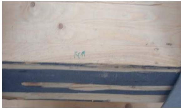
Figure 19 : Delamination between CFRP layers below beam P2 mid-span.
