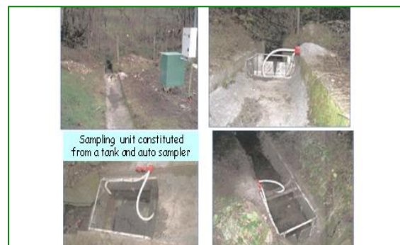
Figure 11 Water pollutant monitoring system instrumentation details on motorway A7
