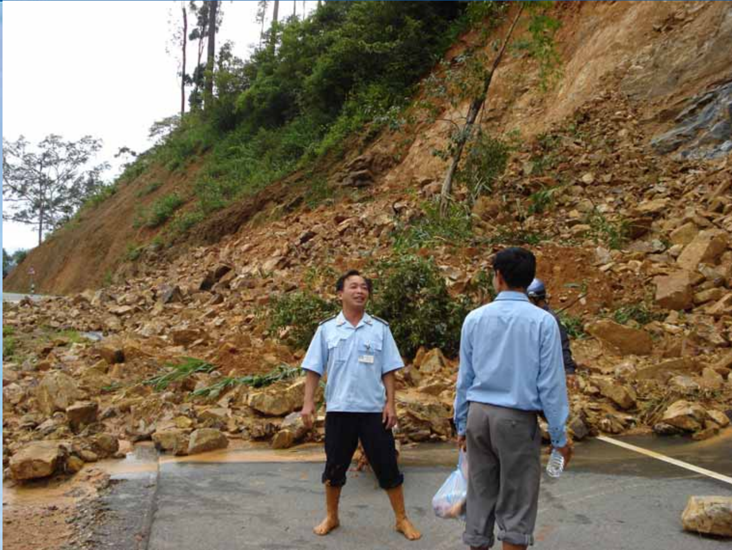
Typical above-road failure
