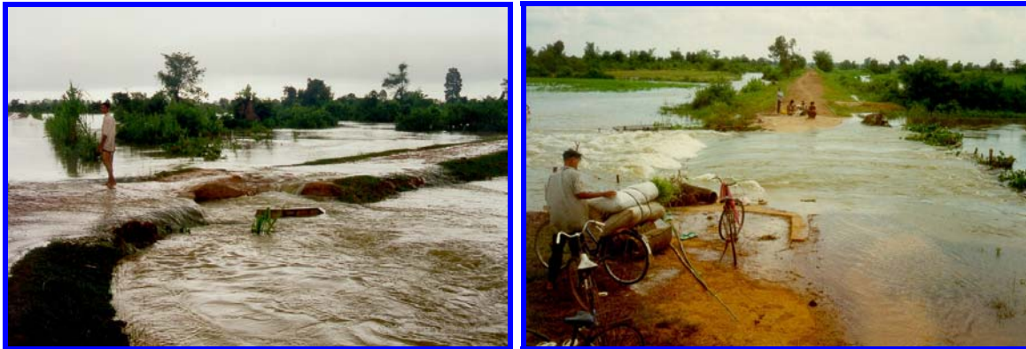
Images 1 & 2: Roads damaged by flood
