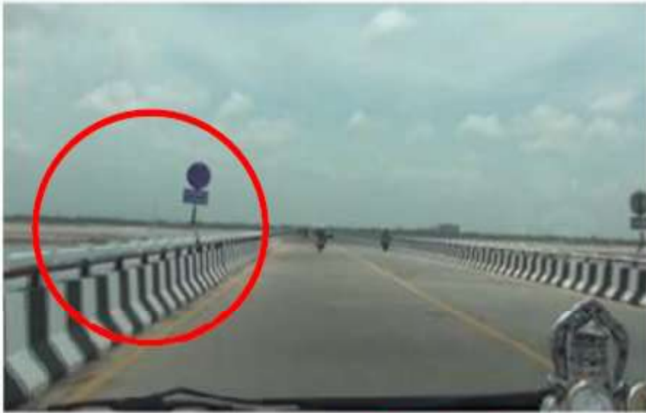
Photo 6.144 At Km.21/700, Reflective Stickers on Parapets of Major bridge is required, place the speed sign, no over taking sign at 500 meters distance as per IRC :65 (2012)
