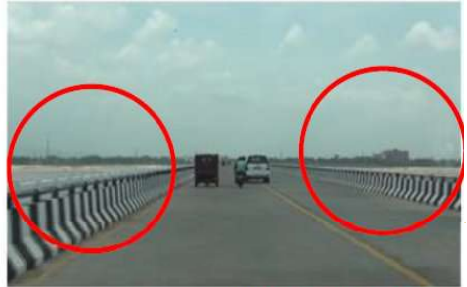
Photo 6.145 At Km.21/800, Reflective Stickers on Parapets of Major bridge is required, place the speed sign, no over taking sign at 500 meters distance as per IRC :65 (2012)
