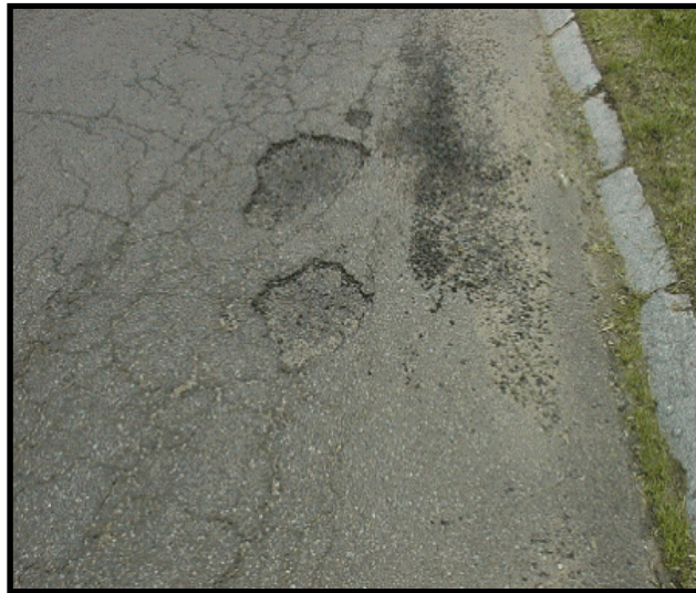
Moisture induced damage
