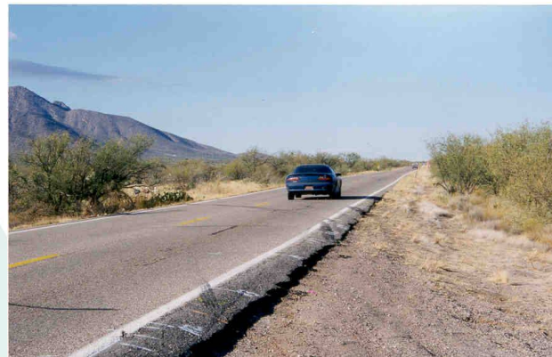
Condition 2. Contiguous drop-off in excess of 2 inches stretching for about 1/3-mile along the roadway. Vehicle may be damaged when pulling onto the shoulder
