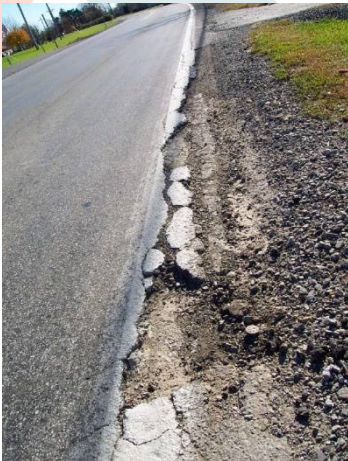
Condition 3. Contiguous drop-off in excess of 2 inches stretching for less than 1/4-mile along the roadway. Noticeable bump when pulling onto the shoulder
