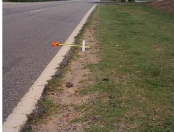
Condition 4. Contiguous drop-off in excess of 2 inches stretching for only about 500 feet along the roadway. Travelers may experience a moderate bump when they leave the paved surface
