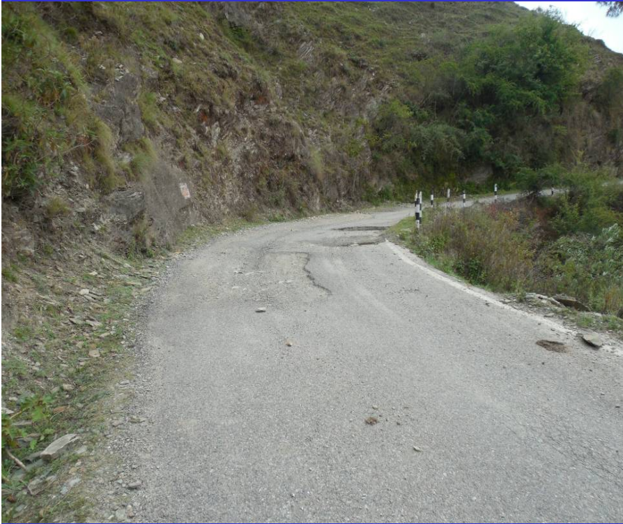
Absence of Drain can Erode the Road
