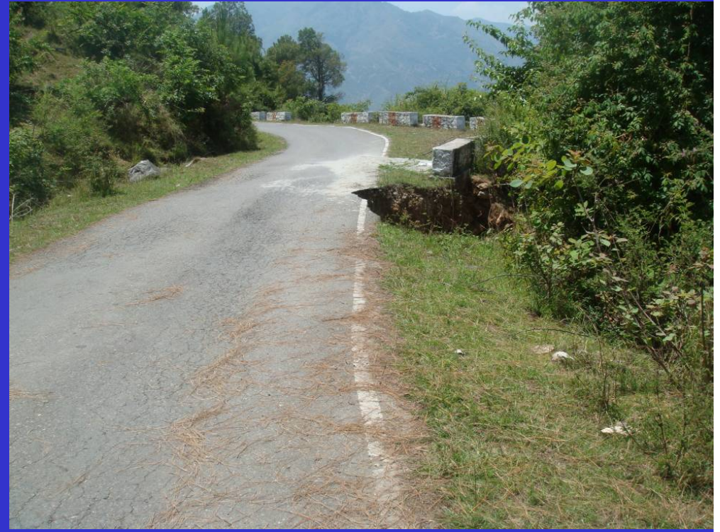
Blocked Drain can Erode the Road
