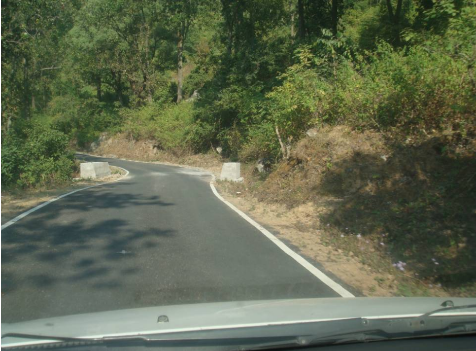
Delineation of the Culvert head walls and trees is essential
