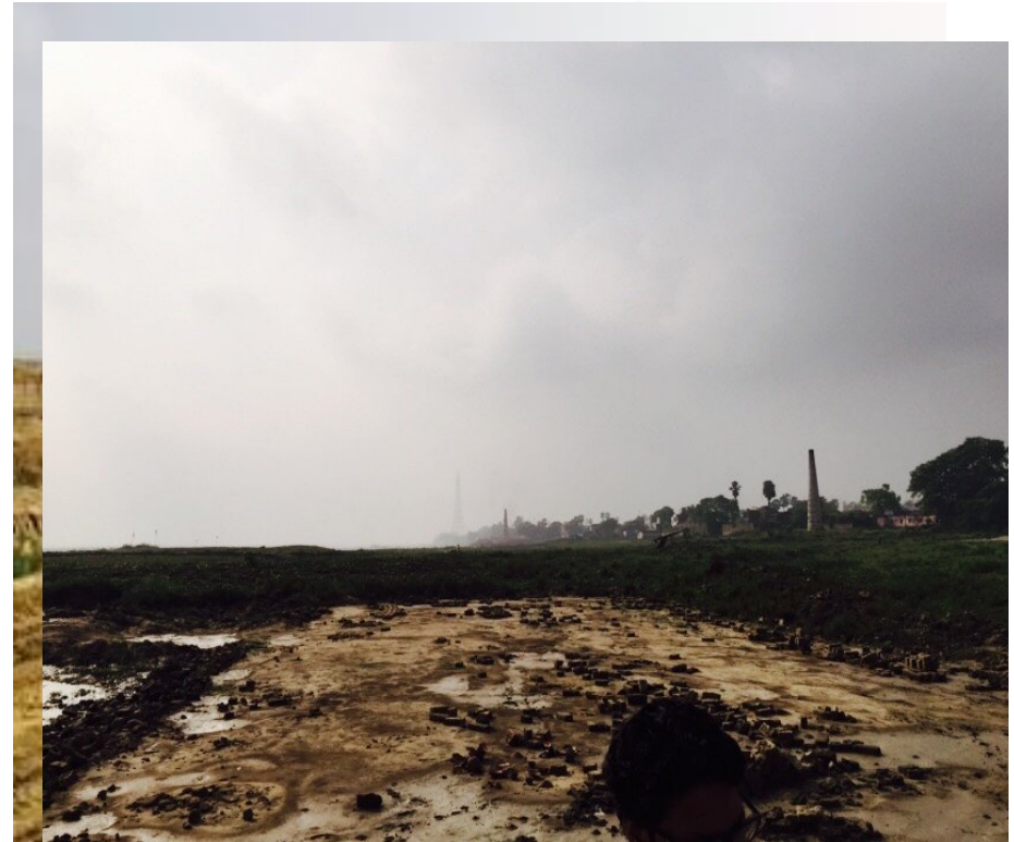
Presence of soft soil in the existing strata of the road embankment
