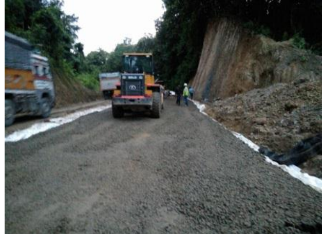
FIGURE 6(d) Pavement without bituminous topping
