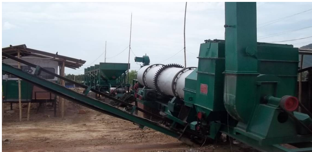
Image-3, Existing HMP
