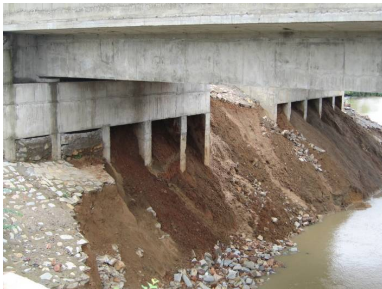
FIGURE 8 Failure of slope of spilling soil
