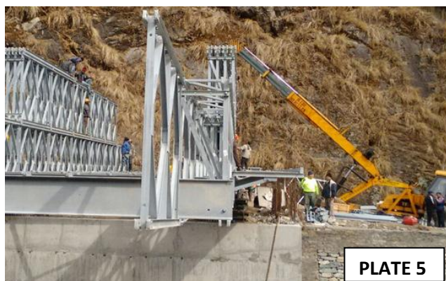
A Quadruple Panel Two Storey Truss Bridge being launched, with the launching nose leading.
