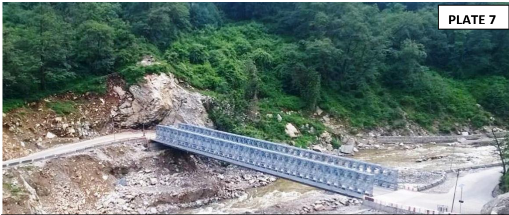
ACROW Bridge at Sonprayag in position, 60m Span, for double lane, 70 R loading, launched in one month with restricted back-space; the first of its kind in India.
