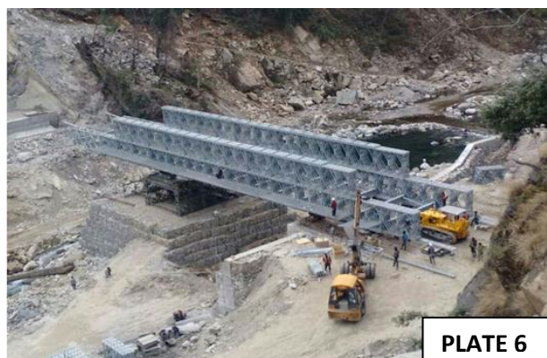
Problem of back space overcome with an intermediate pier and suitable counter weight.
