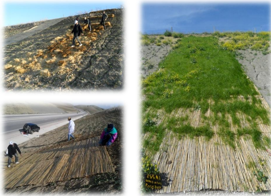
FIGURE 4 Photos of work and results of soil fixation by biological engineering techniques on Moroccan highways
