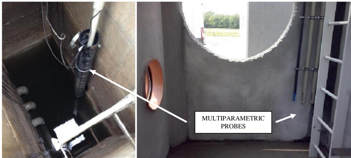
FIGURE 11 Details of different multiparametric probes installation
