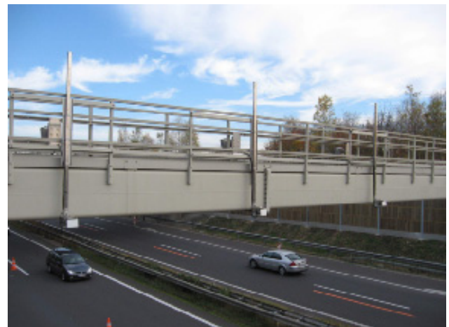
Figure: Overhead traffic sensors installed at a toll station gantry (ASFINAG)
