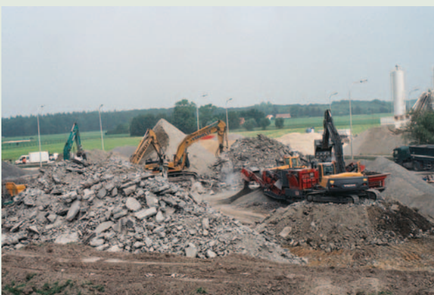
Recycling of materials after road demolition is a key factor when assessing the sustainability of a road
