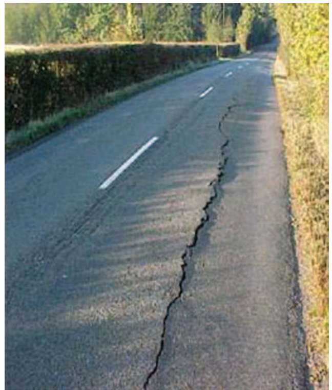
Road deterioration caused by temperature and rainfall extremes
