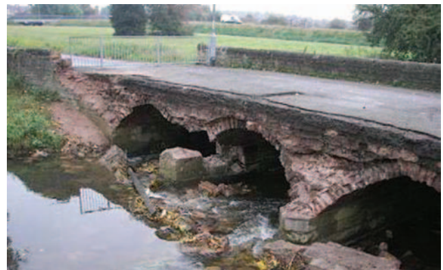
Bridge damage following a flooding event
