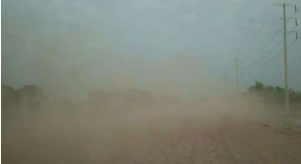
Dust from road during construction
