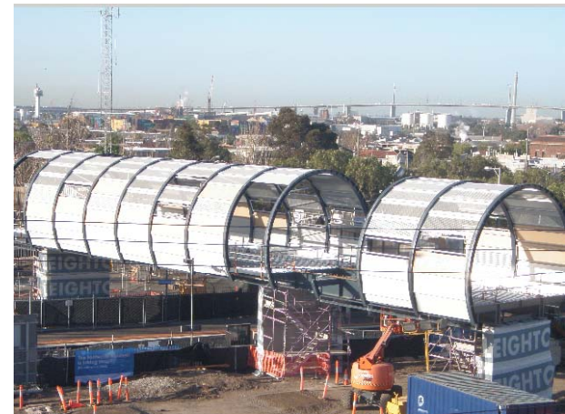
The images above show the construction of the Footbridge as of 14 September 2009.
