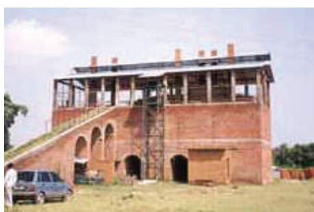
Vertical Shaft Kiln
