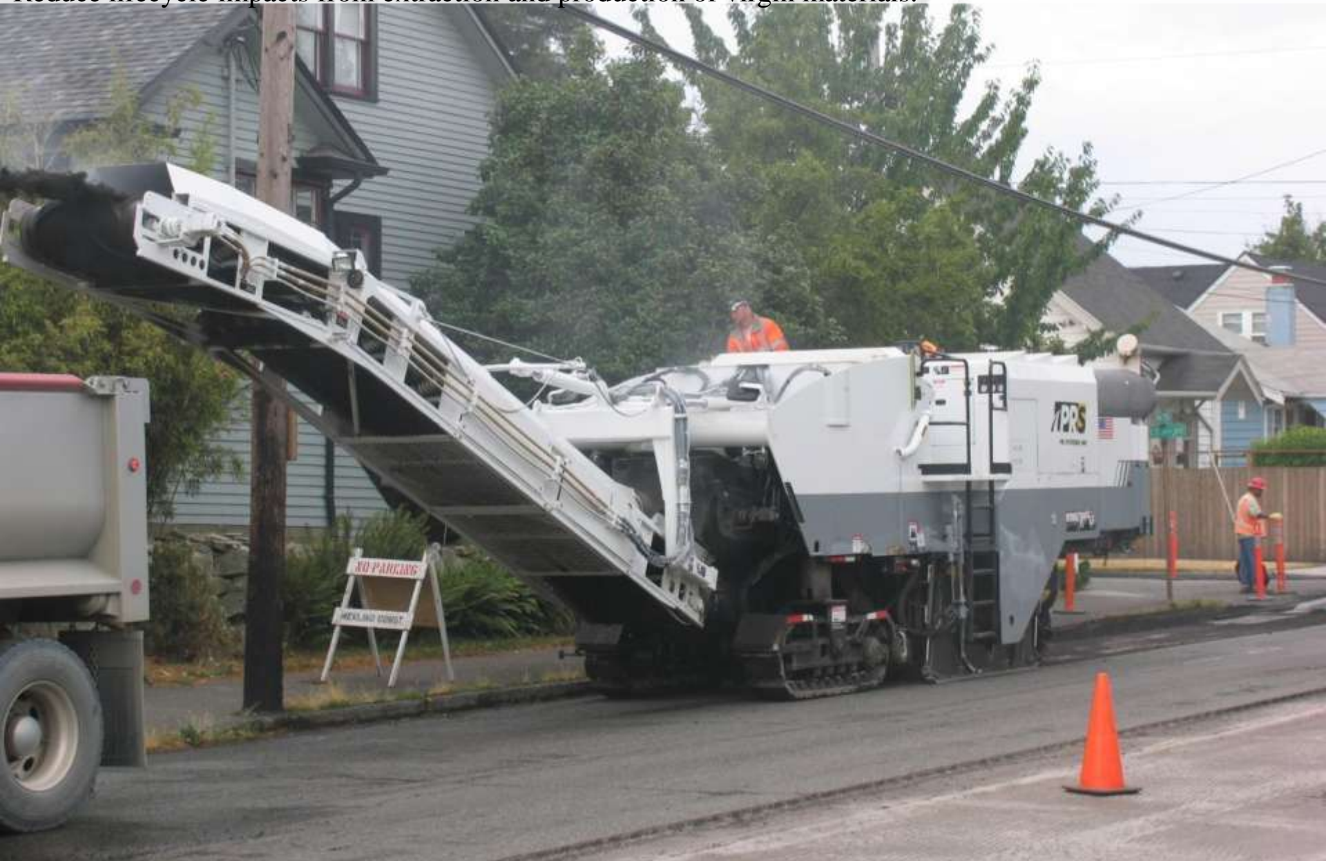
Milling up existing HMA surface, N 75 th Street, Seattle, Washington, United States
