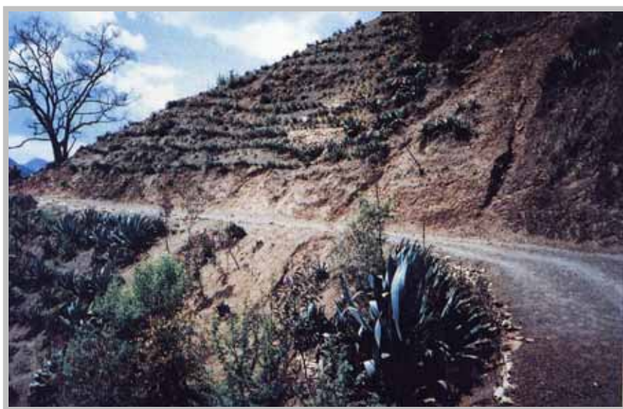
Photo 4817/7 – Palpa, March 1996 Bio-engineering slope stabilisation with Agave along the Banstari – Jhadewa road
