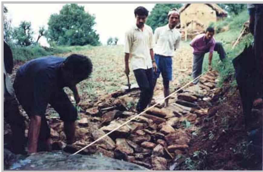
Photo 1128/24 – Lamjung, May 1998 Construction of stone wall and work measurement along Karaputar – Salme Bhanjyang road
