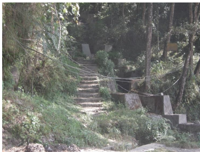
Photo 15.13: Stairs to be strengthened
