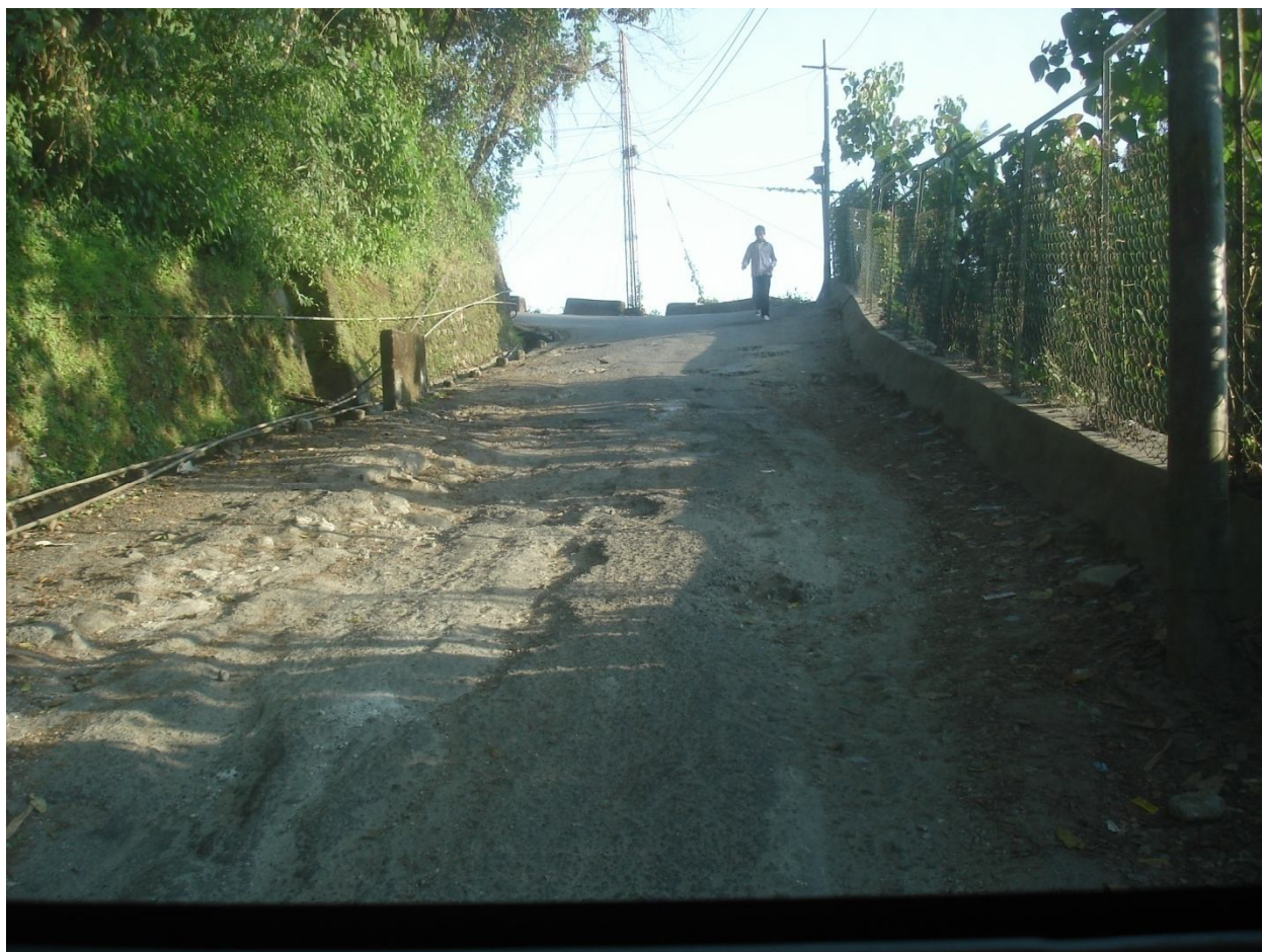
Photo 15.19: Poor Condition of Existing Roads
