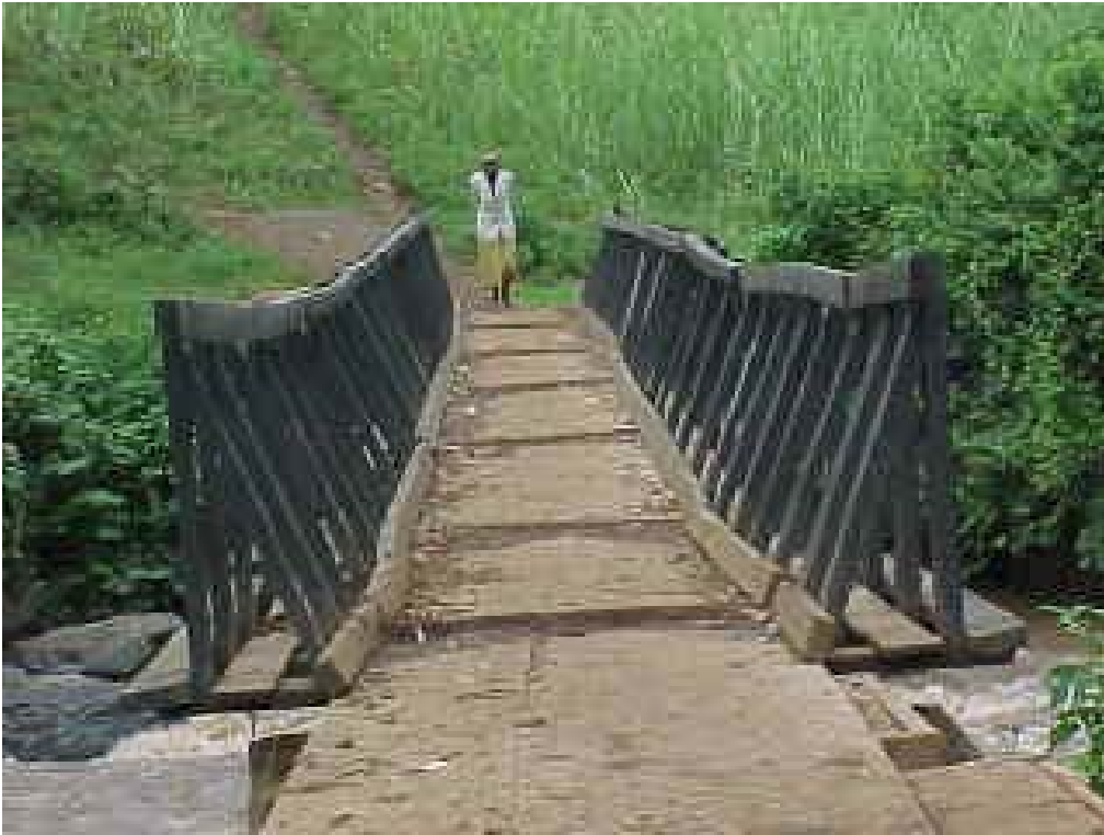
Figure C1: Footbridge Using a Scrap Truck Chassis for the Beams Supporting the Deck
