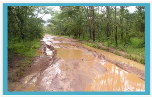
A poor rural road section in Geita District, Tanzania
