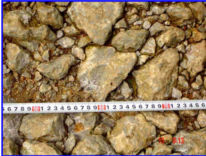
II-A. Eroded Non-Graded Crushed Stone Material. Lau Cai
