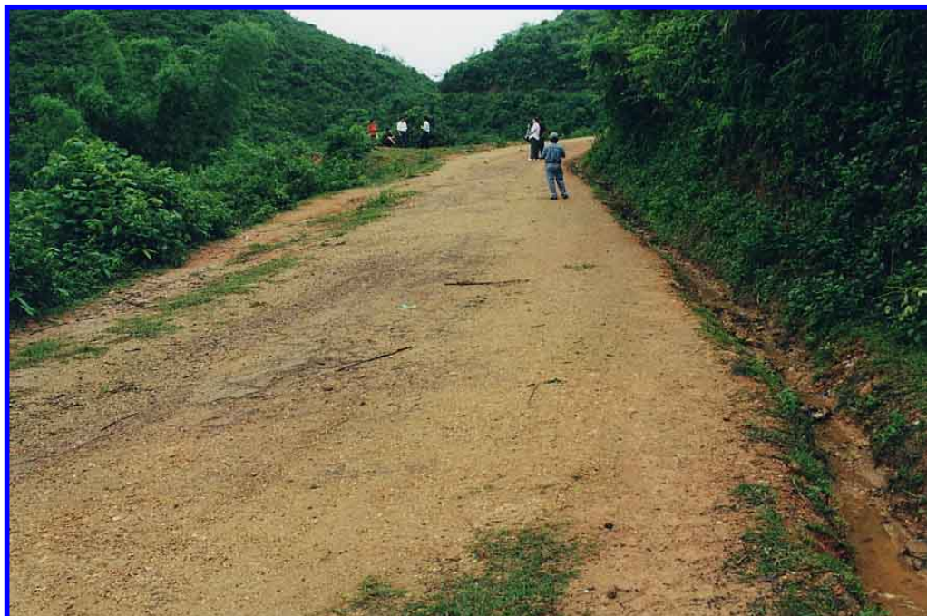
Photographs V : Gravel eroded within 1 year on steep gradient. However underlying material is stronger, suggesting that an Engineered Natural Surface or other use of the insitu material would have been more appropriate
