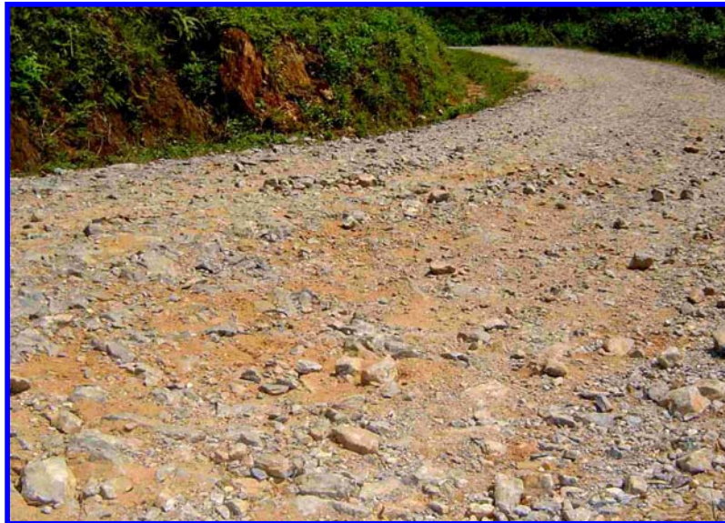
II-B Road Surface Erosion of Non-Graded Crushed Stone Material. Lau Cai
