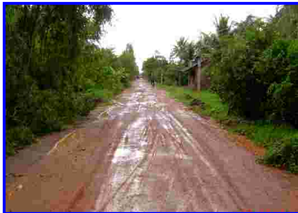
Photographs III : Impeded Run-off and Poor Side Drainage
