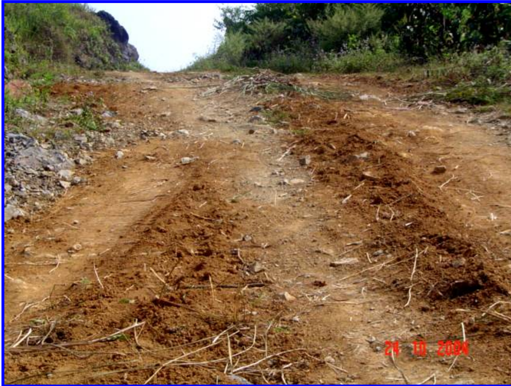
Photograph IV : Inappropriate Material Use for Maintenance
