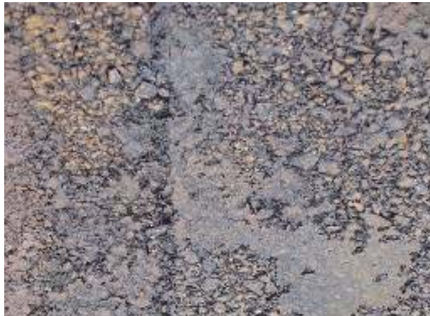
Figure 52: A poorly constructed joint
