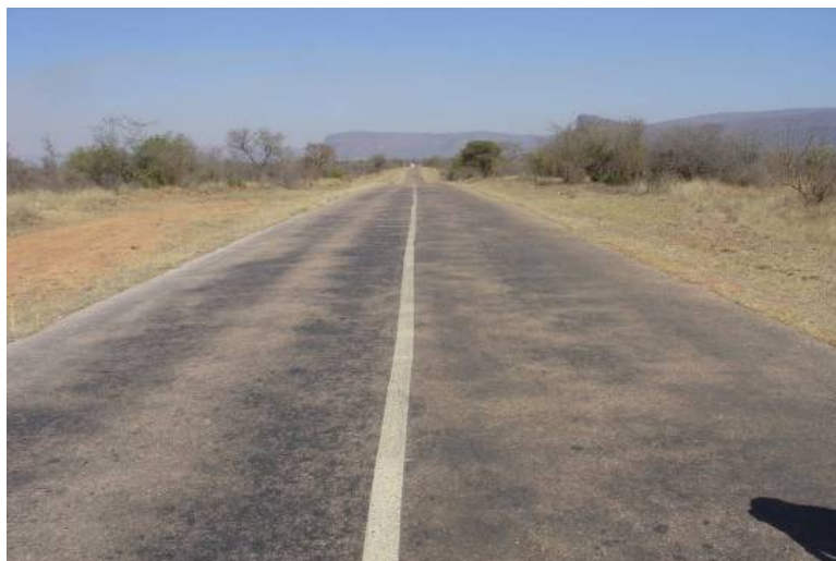
Figure 36: Typical appearance of a single Otta seal after four years in service
