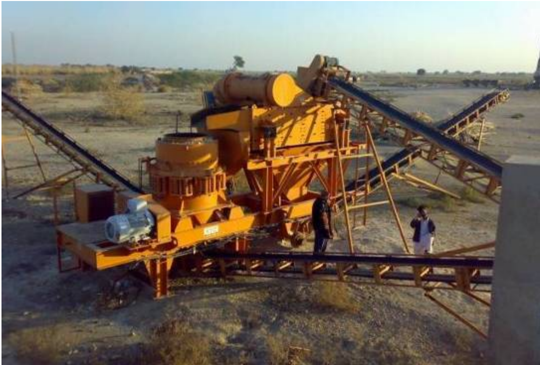
Frame No: 001 Description: Static Crushing Plant
