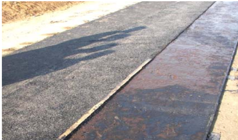
Figure 51: Adjacent strips of asphalt
