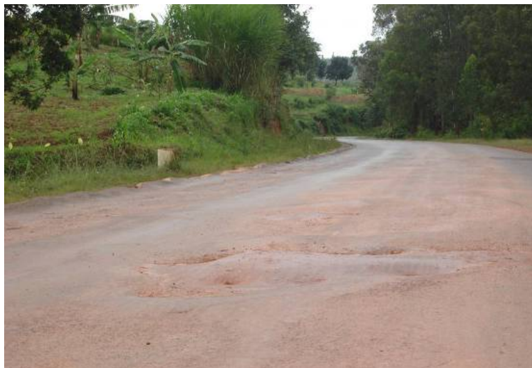
Figure 62: Failed section of road
