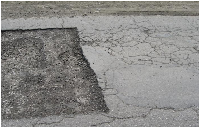
Figure 58: A recently excavated distressed area requiring cleaning, priming and patching
