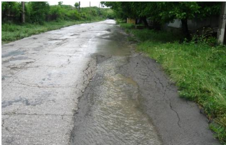
Figure 64: Failed patch and poor drainage
