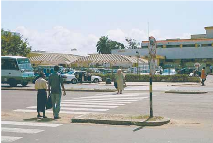
Figure 3.20 Pedestrian crossing opposite hospital entrance with newly installed kerb ramps, cuts in central island and road marking installed as part of the demonstration project in Maputo, Mozambique ( Following the improvements, a huge increase in the proportion of elderly and ambulatory disabled people using the crossing was observed. )
