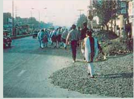
Figure 2.10 Pedestrians are forced to walk past a construction site in India because no facilities for pedestrians are provided by the contractor
