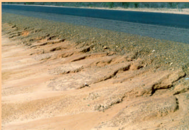
Severe erosion of road side slopes in high rainfall areas.
