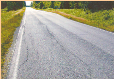
Typical longitudinal cracking and pavement deformation caused by large volumetric changes of an expansive soil subgrade.
